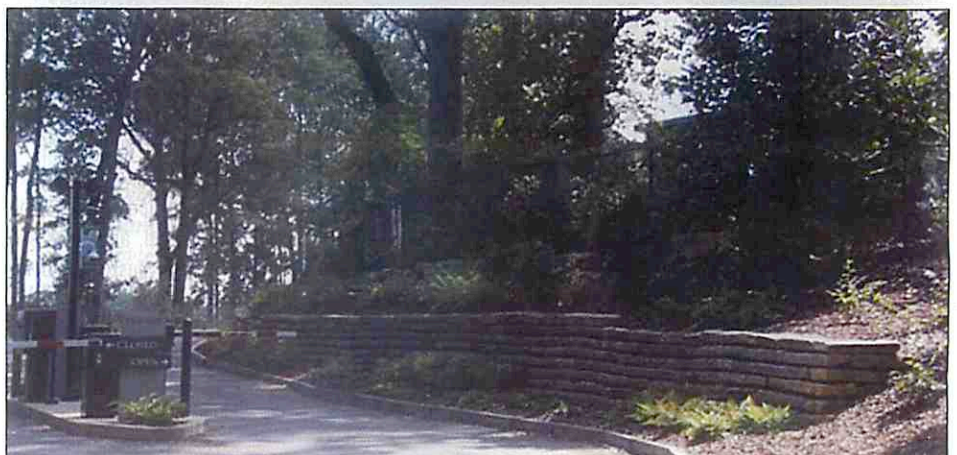
At right, before and after views of a curb wall, with the change in grade for the roadway evident.
