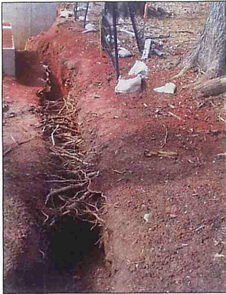
Arboguard used an Air-spade soil excavation tool in conjunction with precision root pruning to prepare the root zones for the installation of new irrigation and utility lines.
